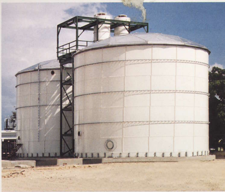
The glass coating on these two Aquastore storage tanks used in treating process wastewater at a brewery in the Dominican Republic is suited to industrial applications.
