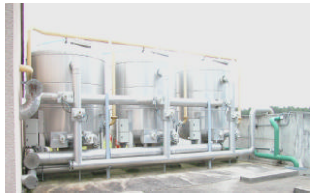
Usine de potabilisation / Drinking water treatment plant, FRANCE
